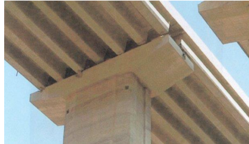
Movement between the piers and the girders of Bolu 1 Viaduct
