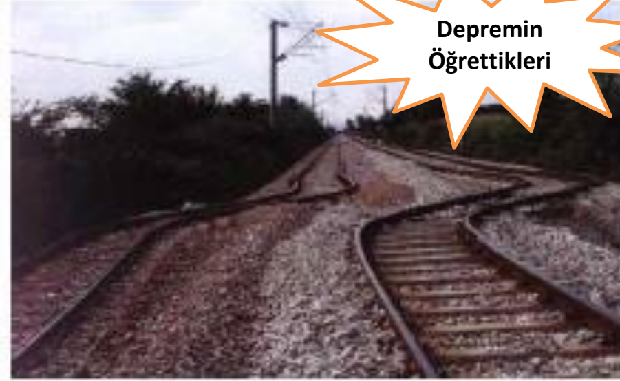
Figure 7.39 Buckled railways near Tepetaria village
