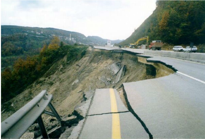
View of the embankment failure (West to East)
