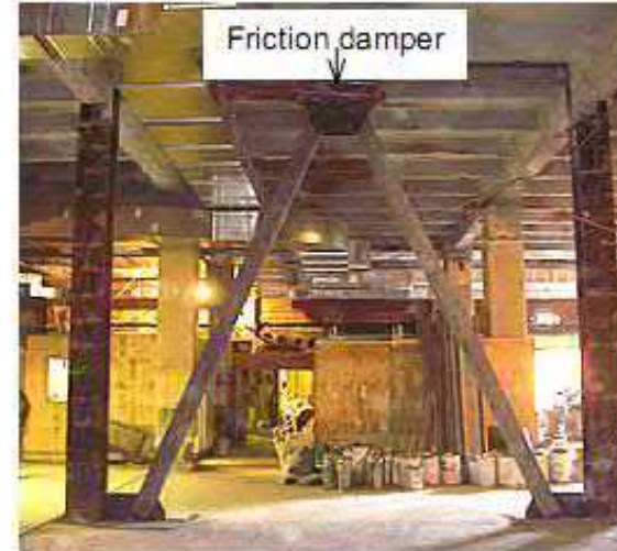
Figure 5. Friction damper at top of chevron brace.
