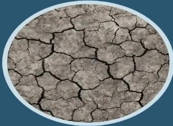
Cracked and deteriorated concrete
