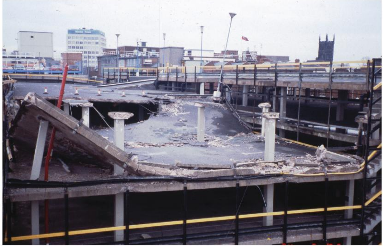
Partial collapse of Pipers Row Car Park triggered by punching shear failure (Wolverhampton, UK, 1997).
